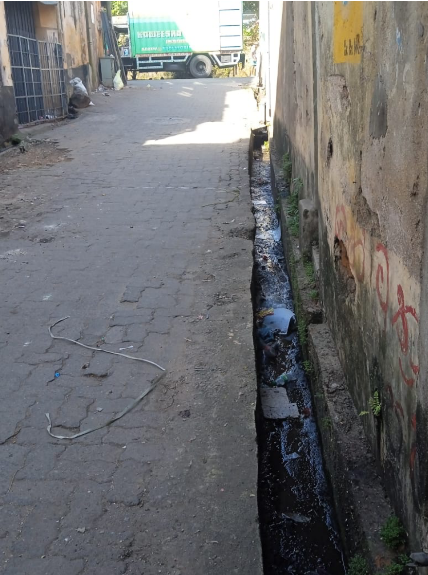
Figure 4: Stormwater drains at Ali Mudukkuwa: centuries-old, narrow, and dilapidated, frequently clogged with solid waste, reflecting the urgent need for restoration and maintenance.
