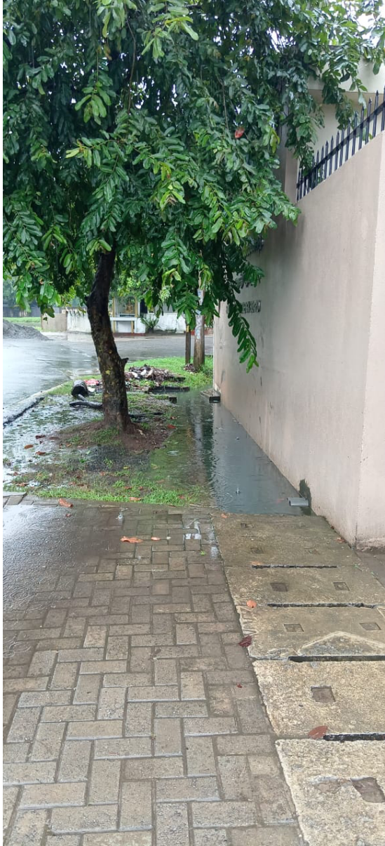
Figure 3: Overflowing Storm Water Drains due to Sedimentation and Solid Waste Clogging
