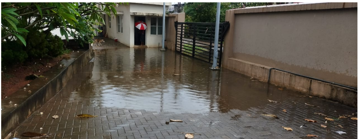
Figure 2: Overflowing drain turns the building entrance into an unpleasant and messy location, highlighting the need for improved drainage solutions.
